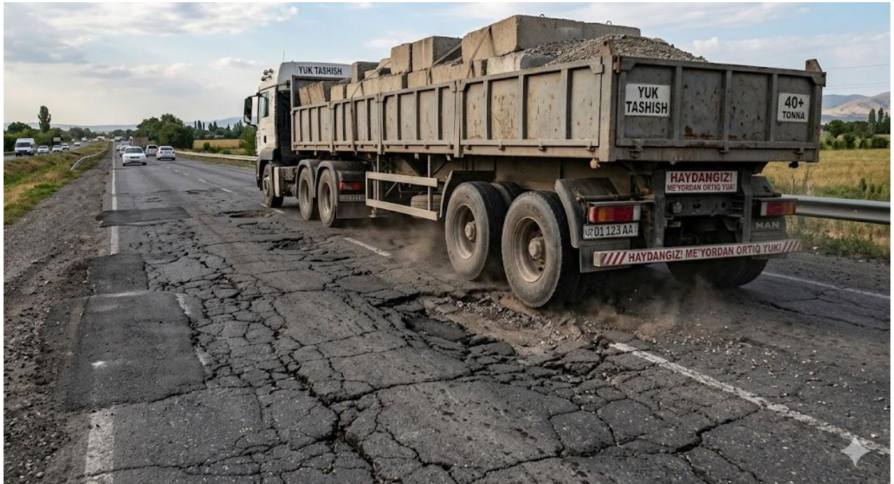
Figure 1. Effect on the road surface during the transportation of heavy goods.
